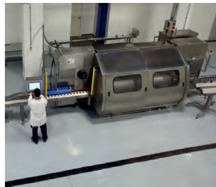
High pressure equipment
