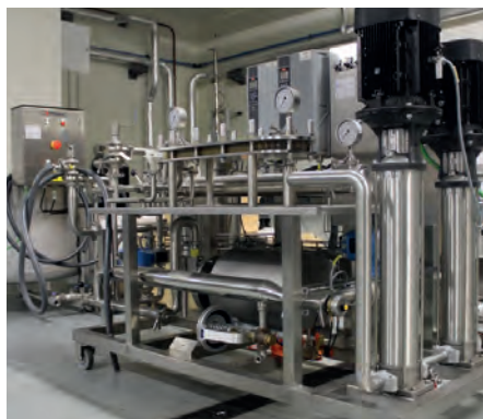
Filtration system with membranes
